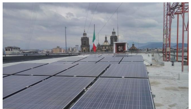
Tigo's long string functionality allowed the PV system to maximize the layout design on each roof.
