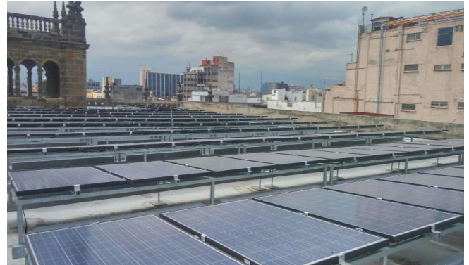
A view of the 116.25kW system carefully mounted on the 500+ year-old roof of the Plaza de la Constitucion.
