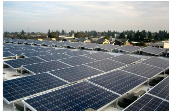
Figure 1: Picture of the commissioned system in Palo Alto, CA
