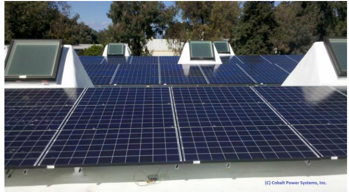
Figure 1: Picture of the commissioned system in Sunnyvale, CA
