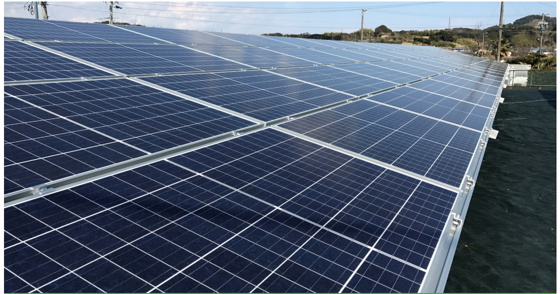
A view of the 76.16kW ground-mount system with 272 modules.
