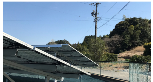
Shade from nearby trees and an electrical pole was mitigated with the addition of 18 TS4-R-M's
