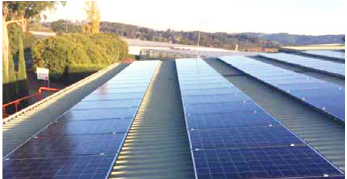
Tigo TS4 optimizers were installed on the back of each Trinasmart module.
