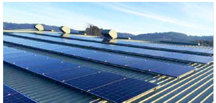
The warehouse cooling rooms may save more than an estimated $13,000 year in electricity costs.
