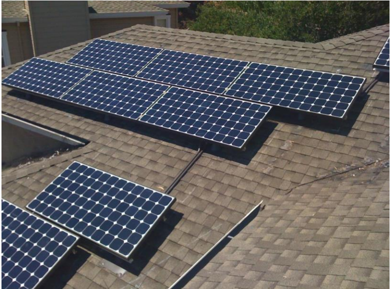
A 4.6kW installation subject only to minor shading.
