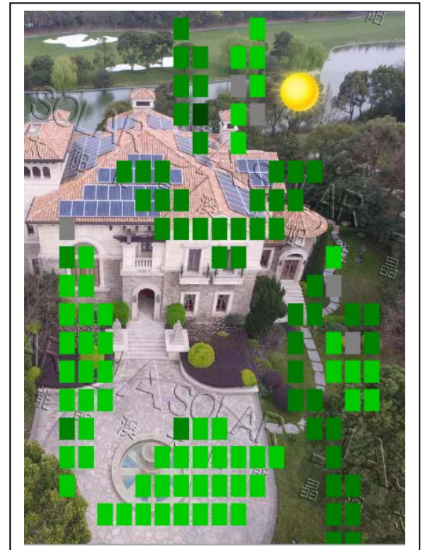
Ingenious and well thought design for this unusual rooftop. Thanks to Tigo® smart modules this difficult layout harvests maximum energy.
